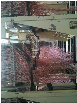
Exchange copper lines
