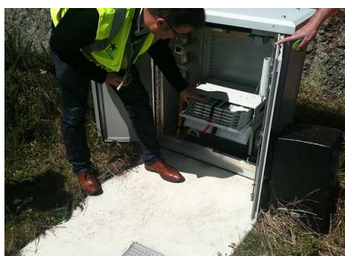
Passive fibre cabinet
