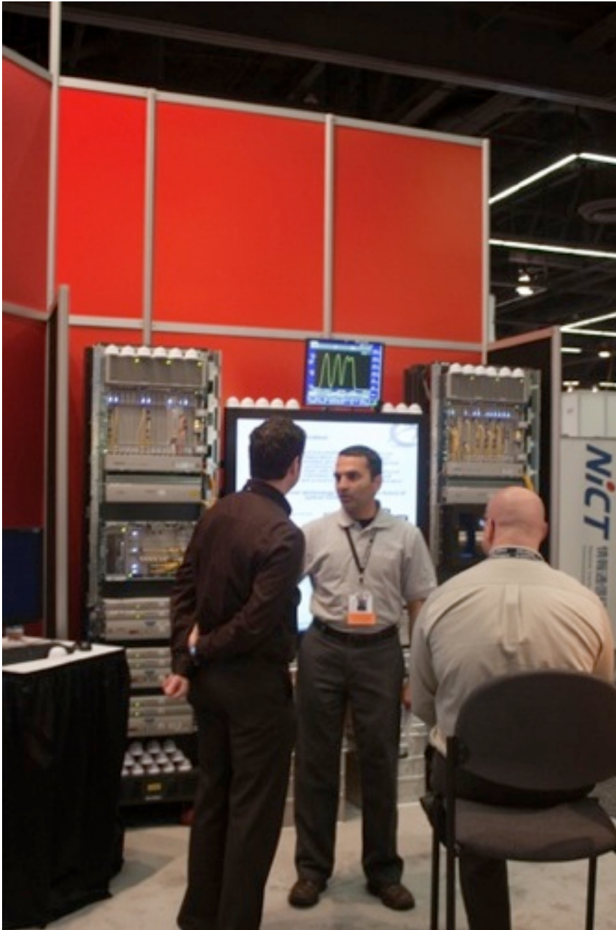
At the Netherlands booth SURFnet was demonstrating how easy it is to upgrade from 10 to 100Gbit/s second in its existing Nortel Common Photonic Layer equipment. Two SURFnet6 nodes were installed interconnected by an artificially long fiber of 1120 km. See the picture on p. 37 below for a close up of the fiber spools seven of which were linked together.
